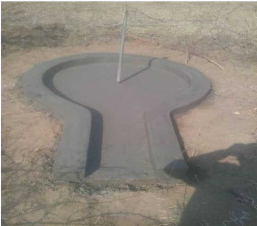
Photo 3: Concrete apron and water oozing out from a recently installed stand pipe
